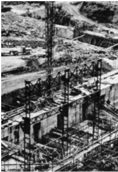
The Balu Chaung hydro-electric project in Burma under construction. Completed in April 1960, resulting in an 80 per cent increase in Burma's installed plant capacity.
